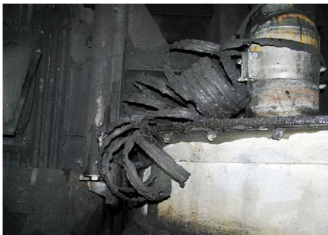
Figure 6. Burned ductwork over T-306
