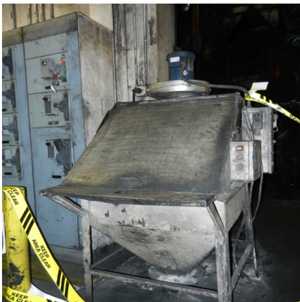
Figure 2. Bag dump station
