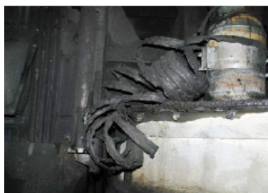
Burned ductwork over T-306
