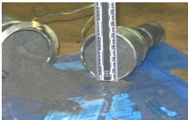
Figure 9. Vacuum cleaning ducts, plugged after less than 2 days of operation
