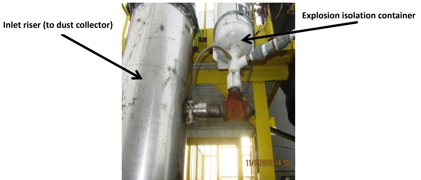
Figure 5. Dust collector inlet with explosion isolation
